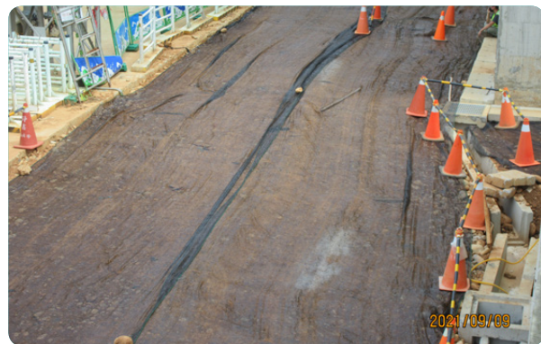
The bare surface of the work area is covered with a dust net to prevent dust.
