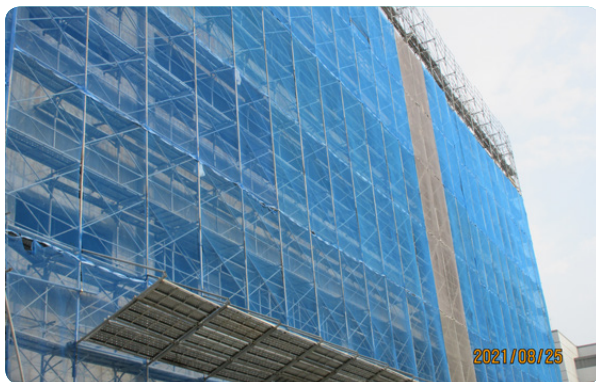
The structure is covered with dust nets in accordance with the regulations.
